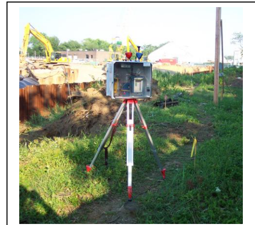
Air Monitoring Equipment
